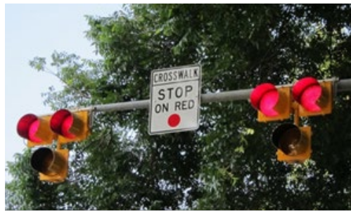
Example of PHBs mounted on a mast arm.
