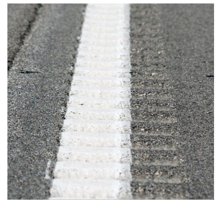
Example of an edge line rumble stripe.
