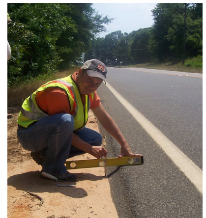
Example of SafetyEdge SM after backfill material settles or erodes.
