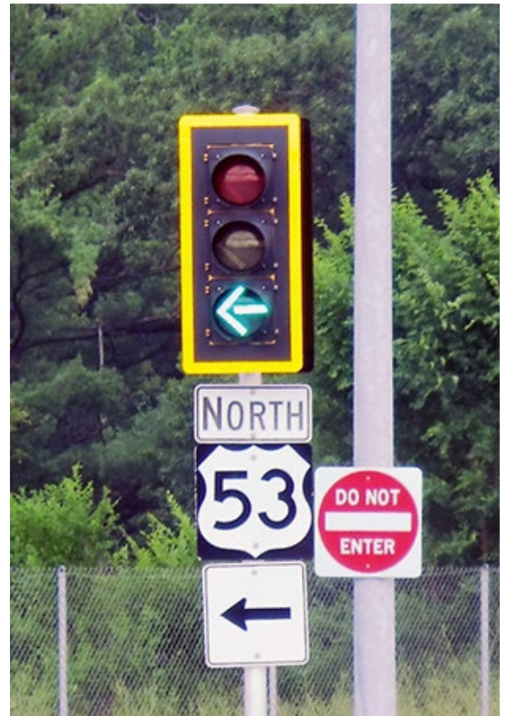
Example of a signal backplate framed with a retroreflective border.
